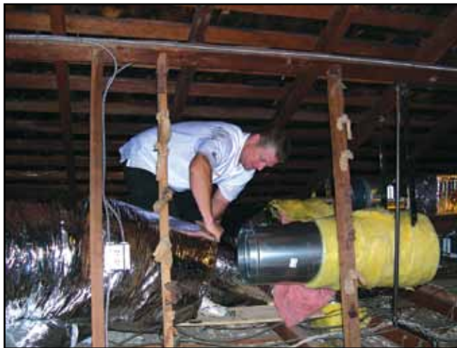
Repairing or replacing leaky ducts can save you a bundle.
